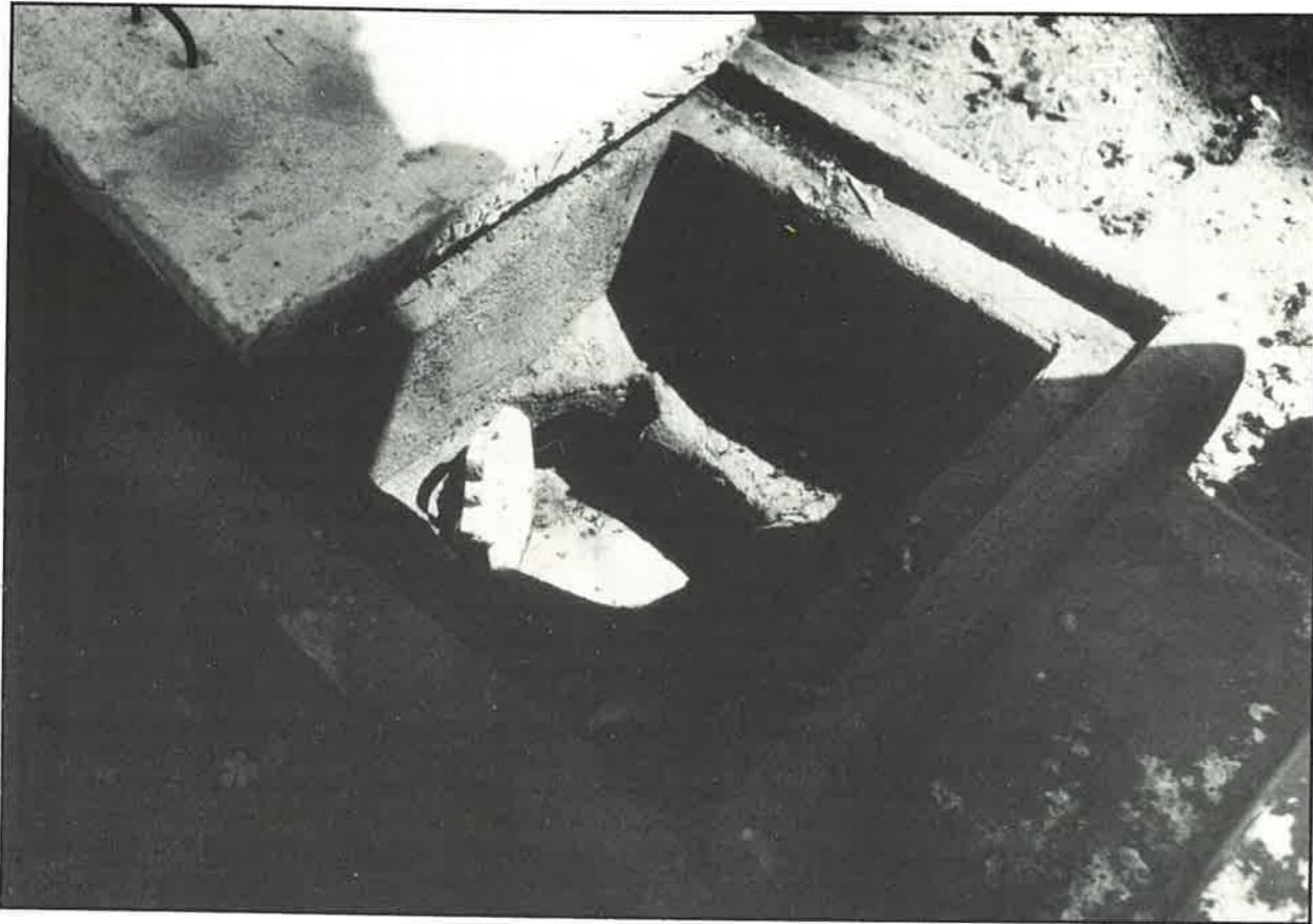
Above: The manhole arrangement for a double pit latrine showing the blocked off entry to the left pit (as viewed)
