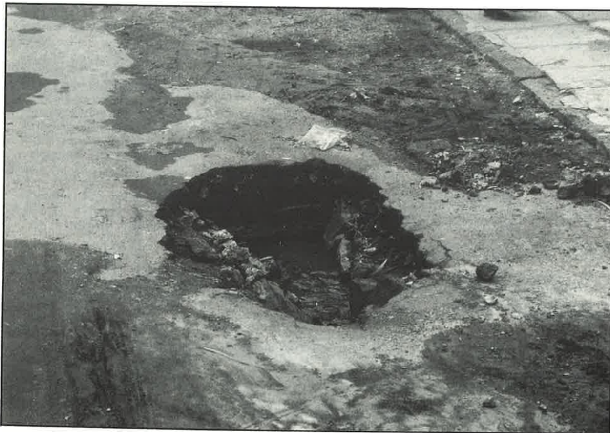
Below: An unrepaired sewer causes the collapse of the roadway
