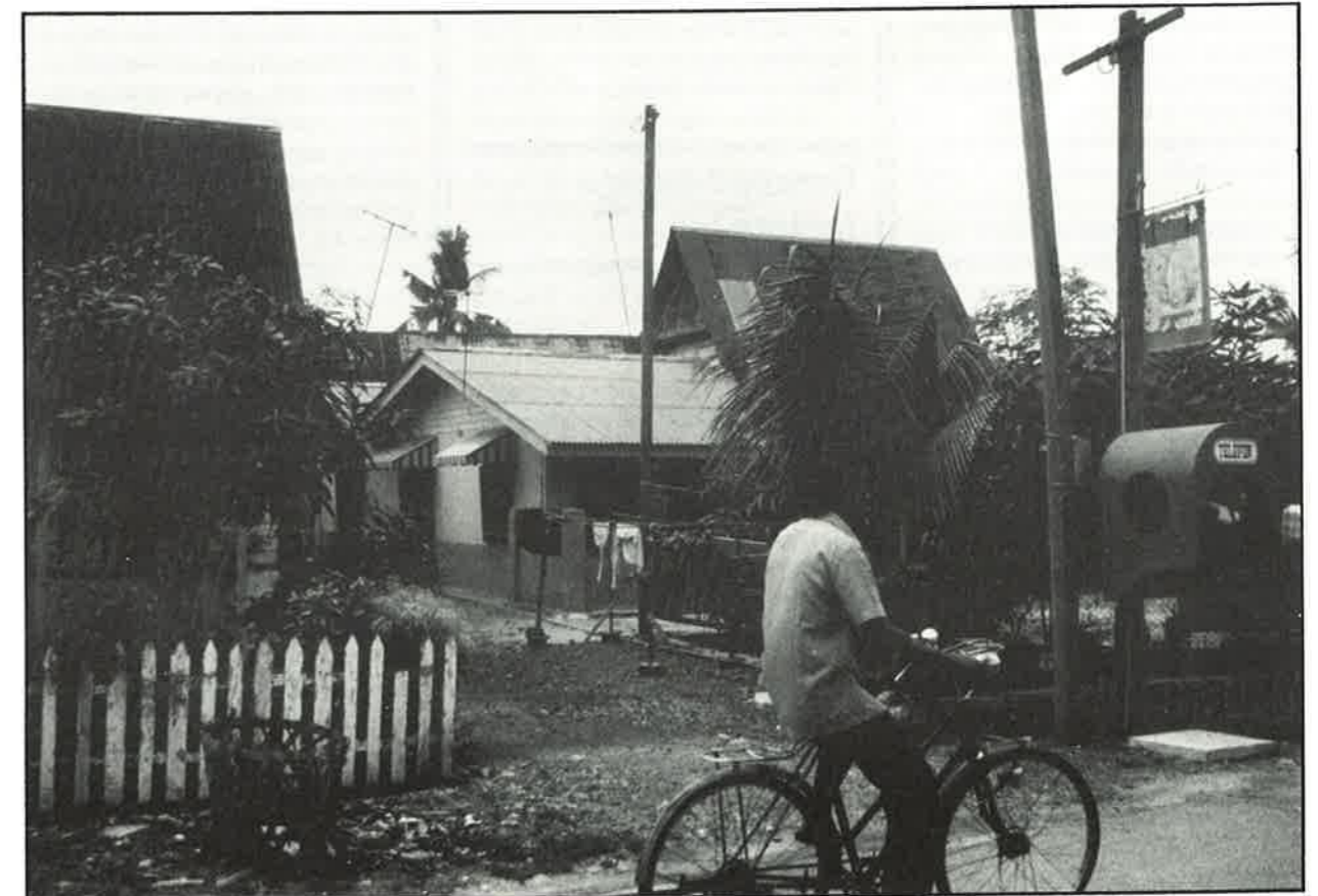
Below: Telephone lines as well as power lines on a low-income housing site
